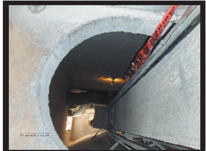
This is the manhole in which my Uncle fell through.
