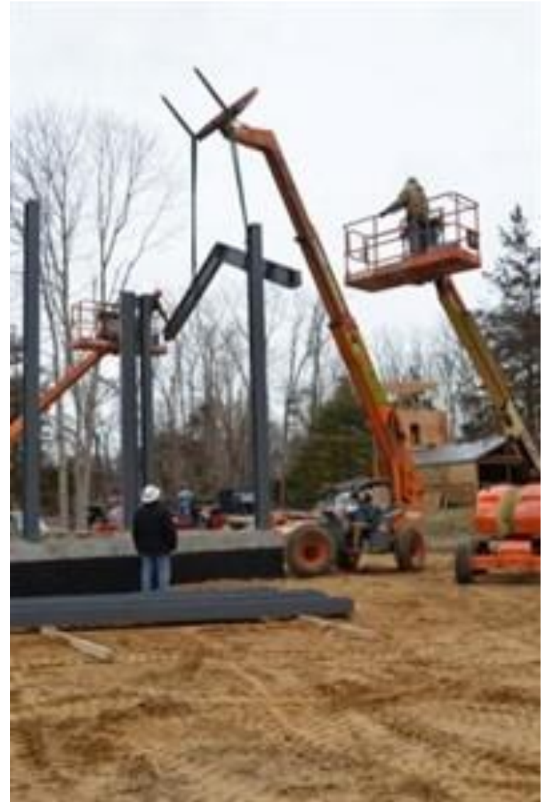
Lifting with a forklift and fiber slings is dangerous.
