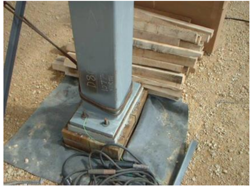
Missing two nuts
